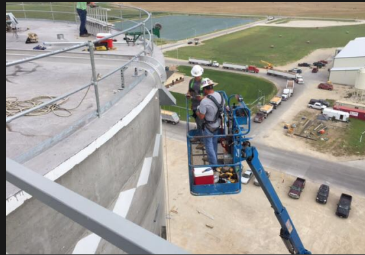
Using the lift to complete some work on grain storage upgrades in Lyons, KS.
